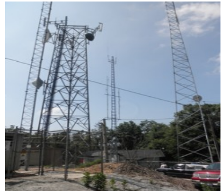
Our KE4RX/r tower with the antennas installed (center)
